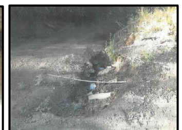
Erosion at the NW
