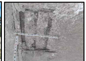
Large Spall in Soffit – Exposing Rebar
